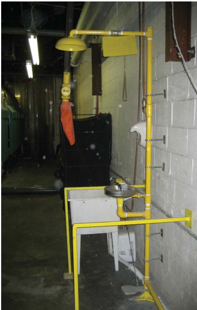
Additional emergency eye wash and shower stations were installed.
